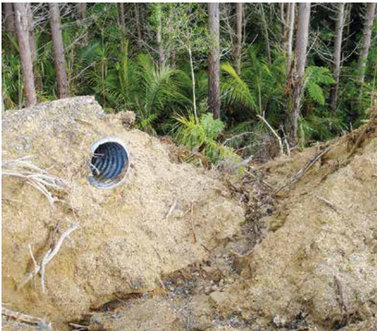
Left: Berm cut-outs can be vulnerable to storm damage because they are compacted fill. Consider armouring, especially when they link to other structures over a fill face, like a culvert sock
