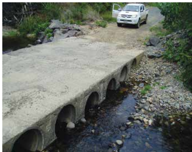
This battery culvert provides for fish passage
