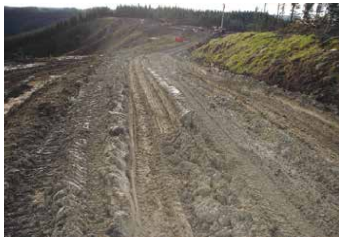
Road rutting creates a safety and maintenance issue
