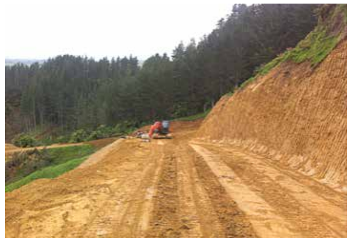
A very high batter with a steep cut slope. While this slope may be susceptible to some slumping and raveling over time, the alternative of cutting the slope back would result in a much greater road prism
