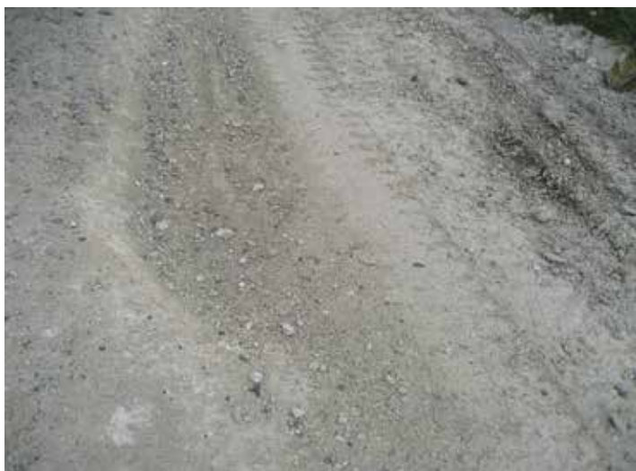
Pavement showing a soft spot
