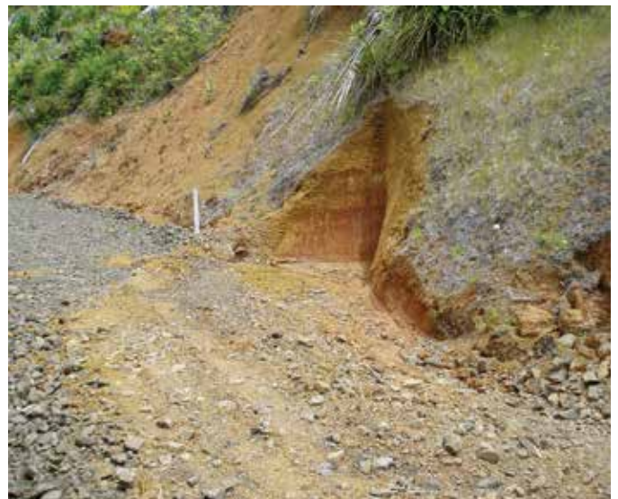
A typical drainage culvert inlet with a sediment trap before it. The trap is deeper than the pipe inlet, and it can easily be cleaned out by an excavator
