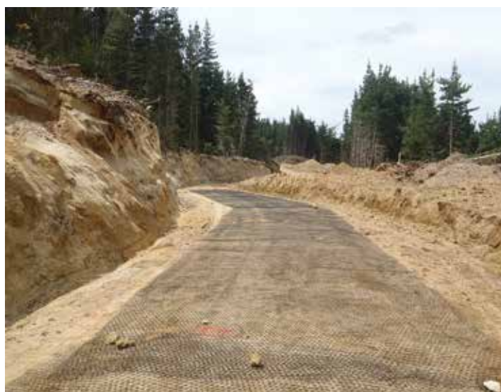
Geogrid laid on a subgrade prior to application of the aggregate layer
