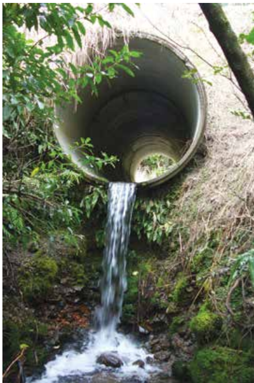
A perched projected culvert eliminates fish passage
