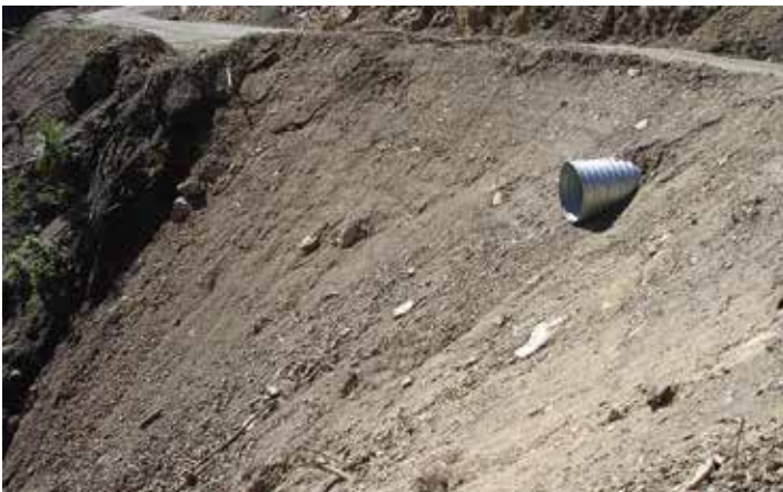
Flumes are needed to reduce fill scour or fill failure. This unprotected outlet will become an issue on the first rain then become an on-going problem
