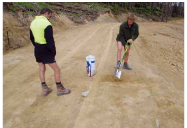
Collecting a soil sample for analysis can provide detailed information about its suitability as an adequate base layer, and can also be used to determine optimal compaction levels
