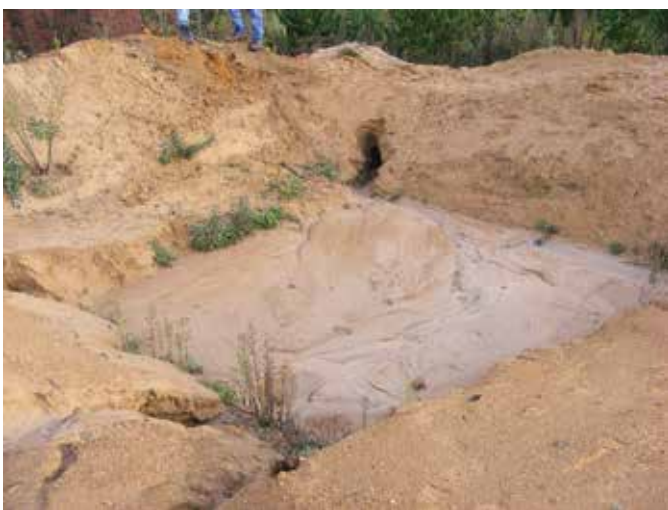
This pond has filled, then the wall has become saturated, and finally the water has sluiced through it
