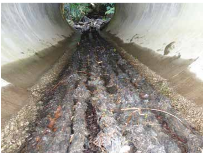
Mussel spat ropes are the most cost-effective solution for fish passage. (Credit: Bruno David, Waikato Regional Council)
