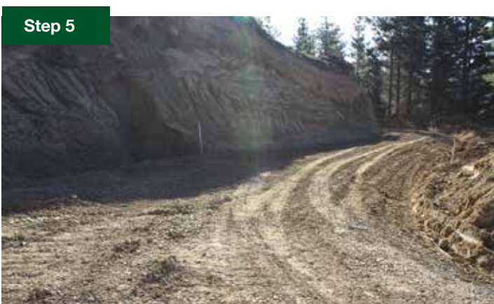
Culvert installation steps: 1. Construct the inlet. 2. Dig the trench at an angle to the road. 3. Bedding the culvert. 4. Compact fill around and over the culvert. 5. The completed culvert with markers
