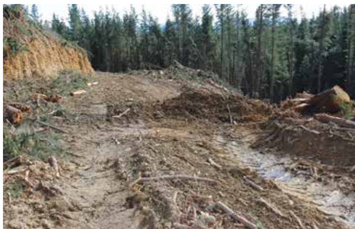
Managing temporary harvesting tracks is not discussed in this Manual, but cut-outs play an important role in track rehabilitation
