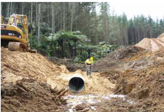
Compacting fill material around a culvert is important to avoid failure in the long term
