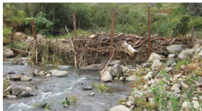
This highly effective debris trap needs to be cleaned to continue to limit slash from going off-site. Know the NES-PF regulations around debris trap maintenance and reporting
