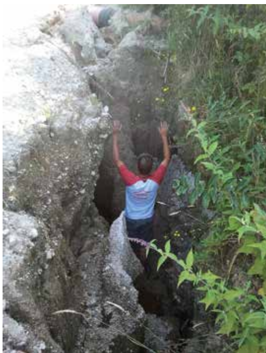
Check ditches for scour. Poor water control maintenance, along with heavy rain and a steep road section, created this bad mix of environmental, health and safety, and infrastructure risk in pumice country
