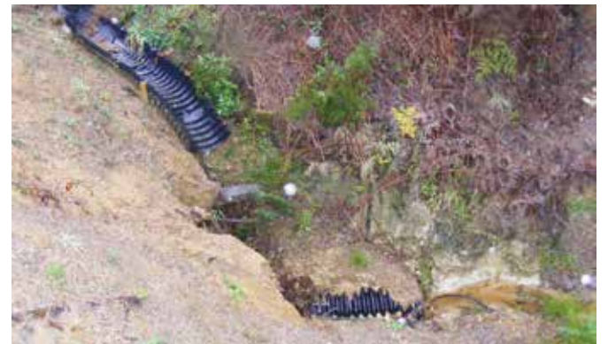
Below: The flume failed because the outlet was not armoured so water undermined and collapsed it
