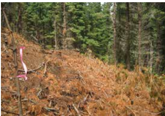
Re-establishing the grade line after road line salvage using taped branches as markers
