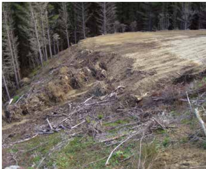
Stumps have been placed on a bench, which is a safe location and one that will not cause environmental issues
