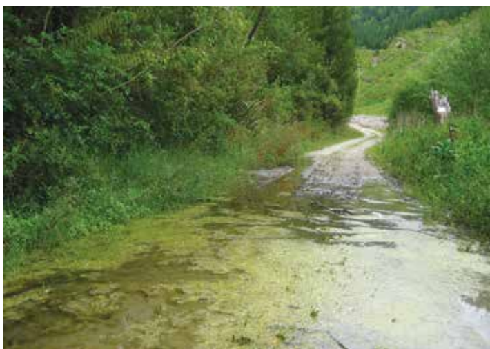
Insufficient ditch depth plus poor shoulder maintenance led to water following the road
